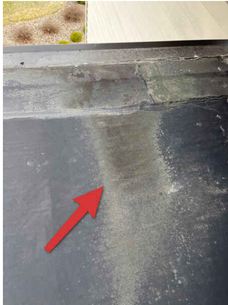
Evidence of ponding on flat roof
