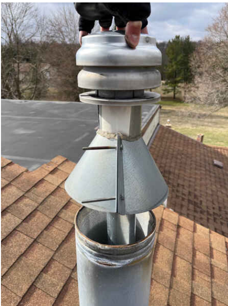
Flue vent loose
