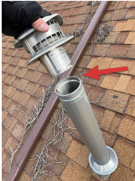
Flue vent not secured
