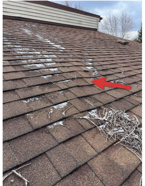
Shingles not laying flat
