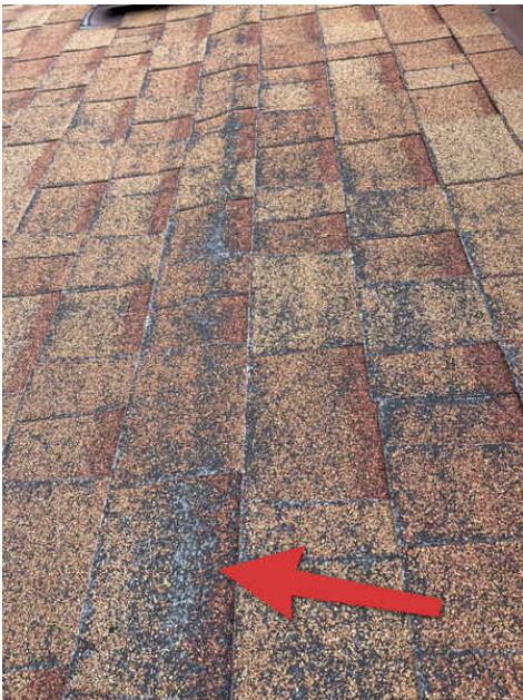
Shingles end of life condition
