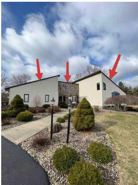
Siding installed diagonally and stone veneer missing weep holes/moisture barrier
