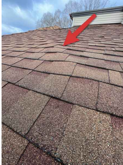
Shingles not laying flat
