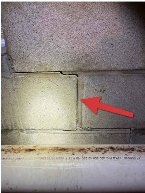
Right - large step crack
