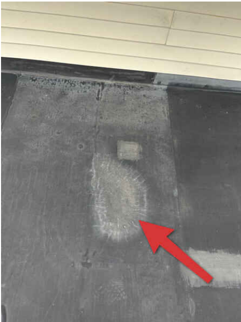
Evidence of ponding on flat roof
