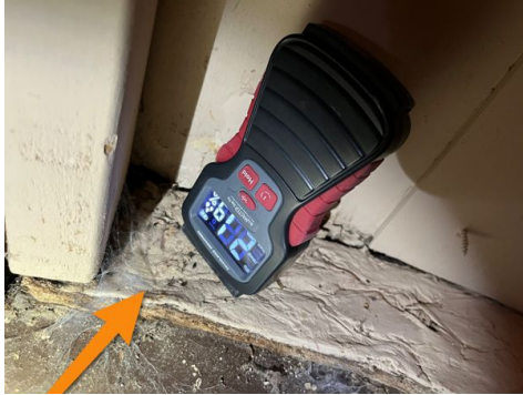
Basement near Goodman furnace
