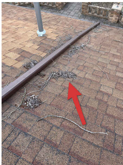
Debris on roof
