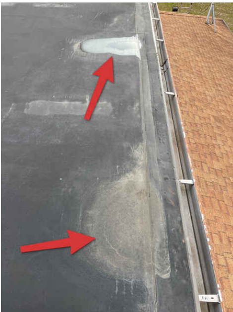
Ponding on flat roof
