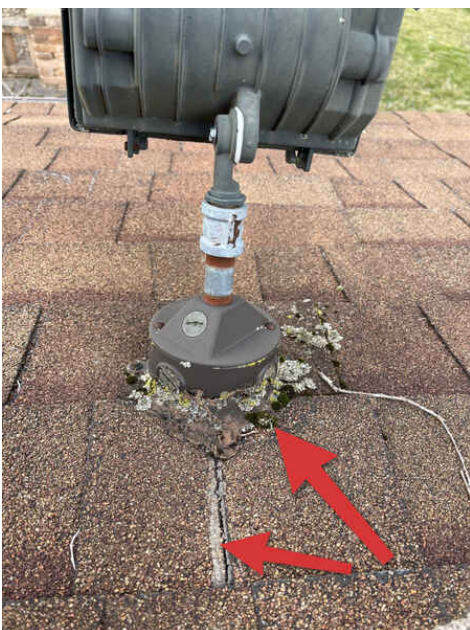
Failing sealant and moss growth
