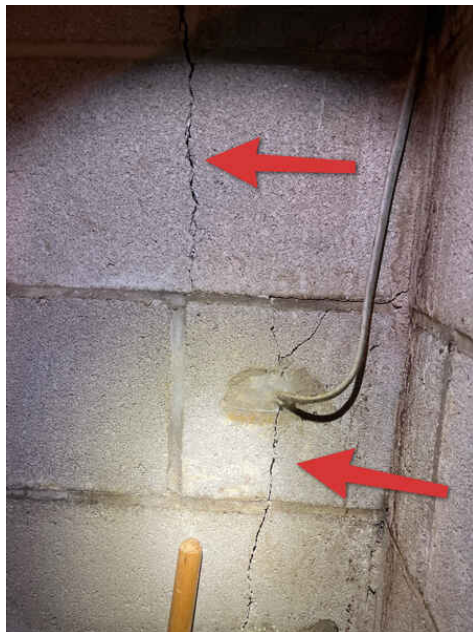
Right - vertical crack
