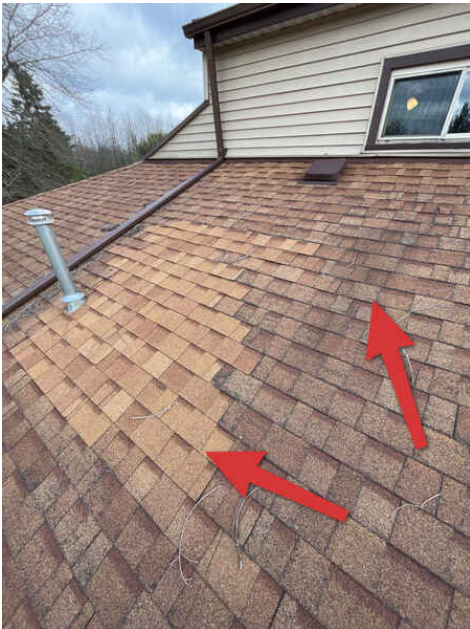
Patching present and major granule loss
