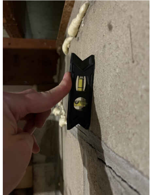
Right - out plumb
