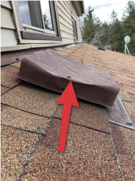
Damaged box vents
