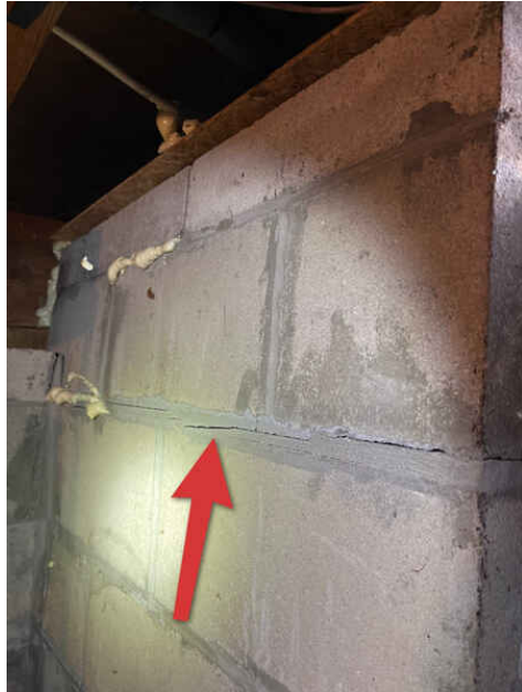
Right - horizontal crack
