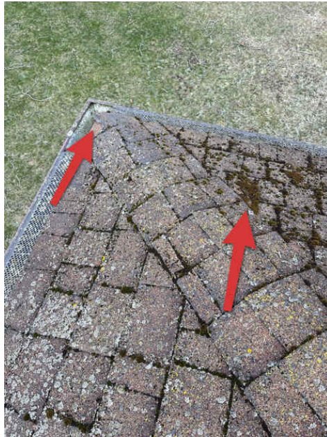
Damaged shingles and moss growth
