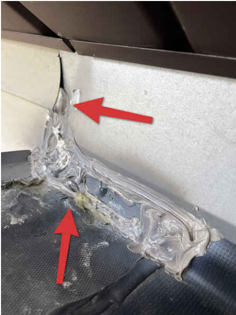
Poorly installed/failing sealant
