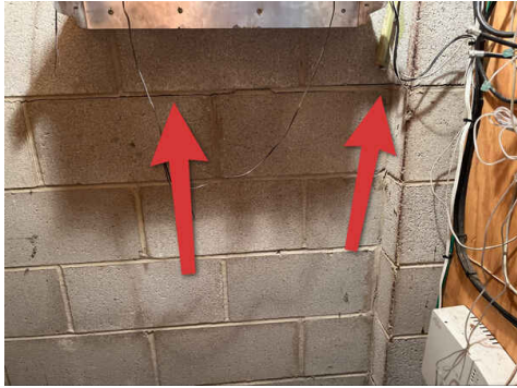
Left - horizontal crack
