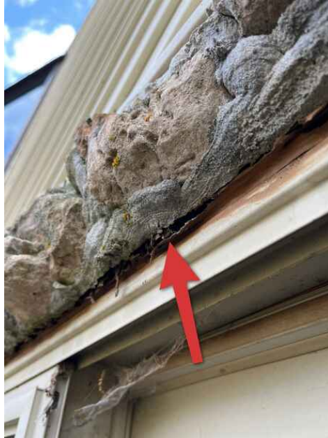
Behind stone veneer - missing moisture barrier
