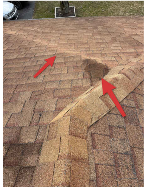
Shingles not laying flat
